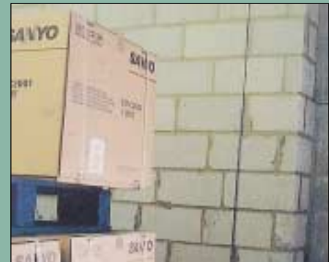
Warehouse protected by WallSecure™ detection system
